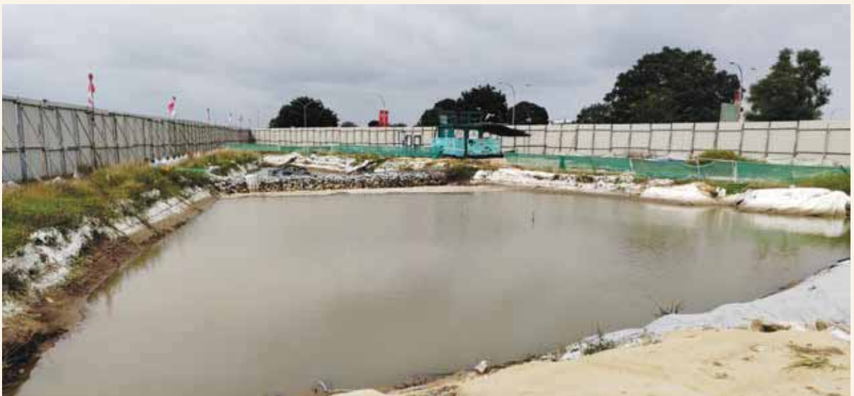
Silt trap at Sultan Ismail Petra Airport
